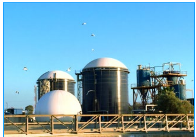
The Hadera wastewater treatment plant
