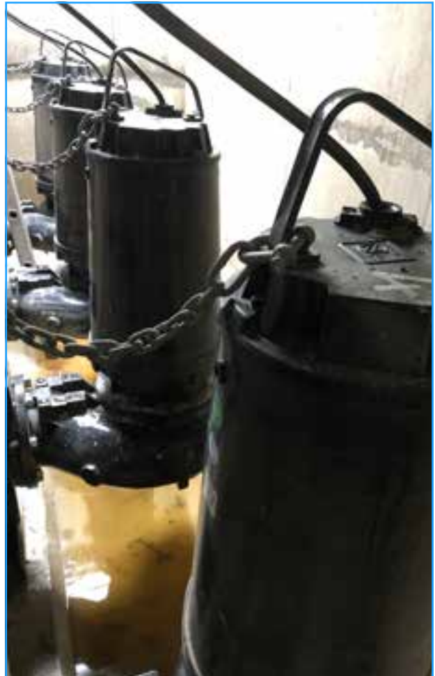
The Uniqa pumping station.
