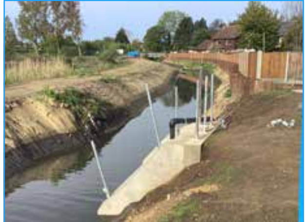
View of part of the project plant.
