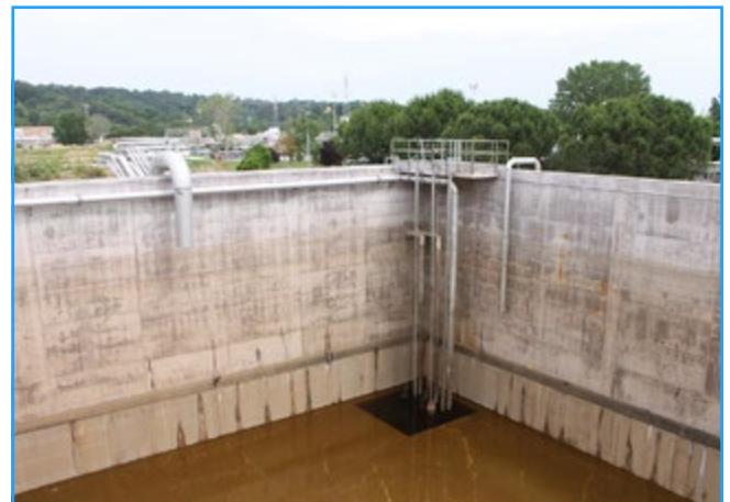
Two tanks of the treatment plant where Zenit machines are installed
