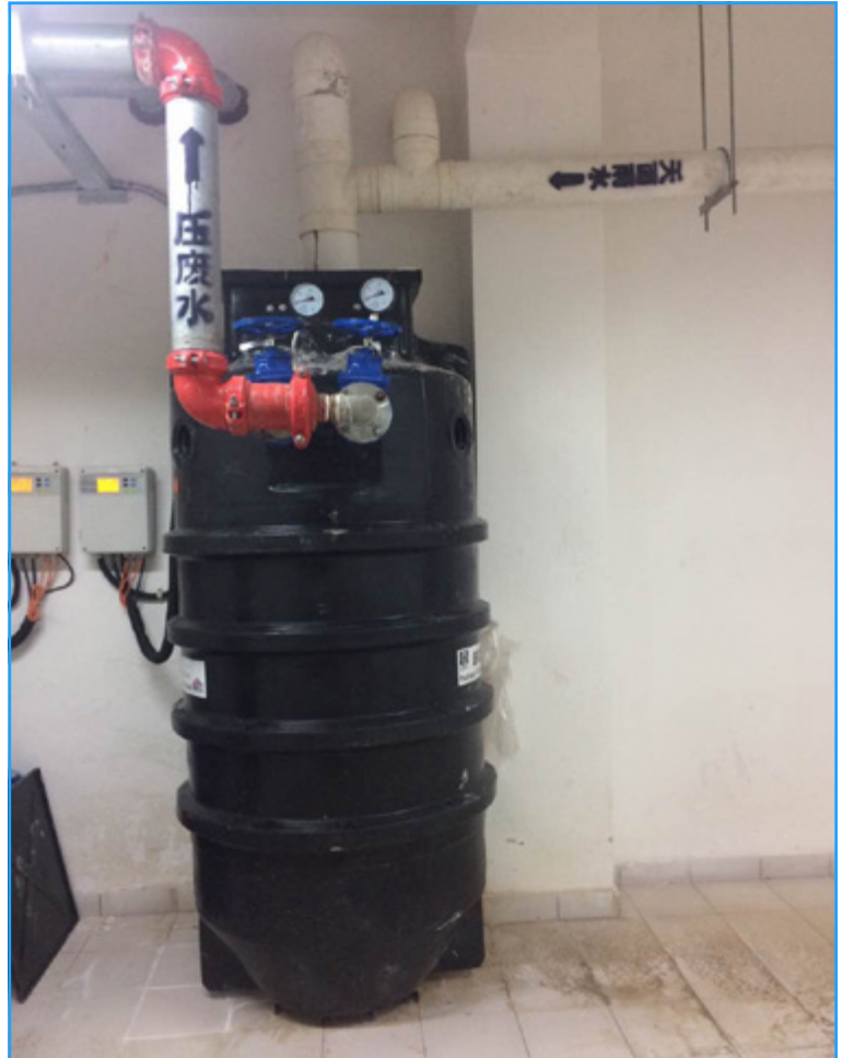
Pumping station operation
