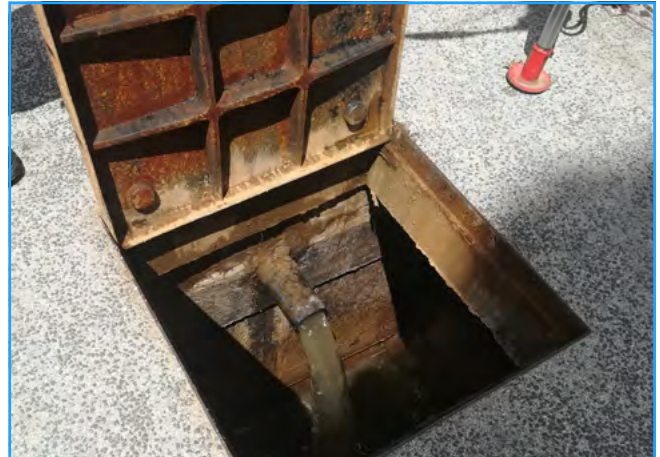
The wastewater to be lifted
