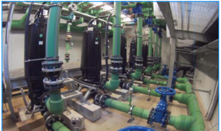
Storm drainage dry chamber
