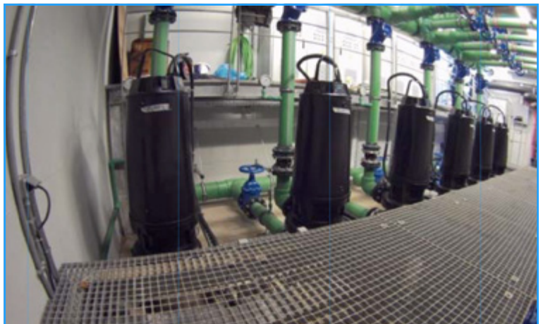
Storm drainage dry chamber
