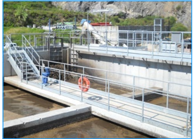
The waste water treatment facility
