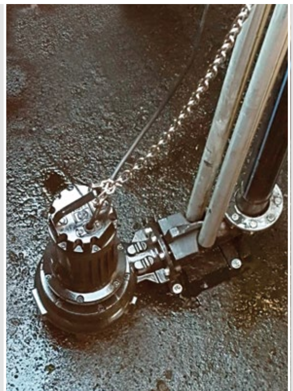
Lifting station pumping rainwater from collection tanks (Italy) Four ZUG V 100B 5.5/4 AW pumps
