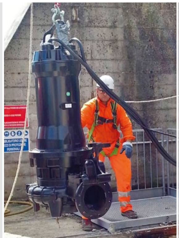
Pumping station for heavily soiled sewage (Italy) Four ZUG CP 250B 45/6 AW pumps
